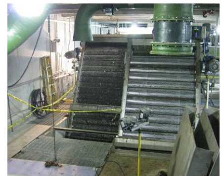
Trash Rake at Treatment Facility
